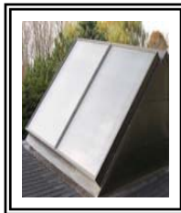
Hot Water Generation
