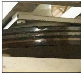
Damaged traction wheel
