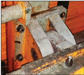
Broken and loose bolts
