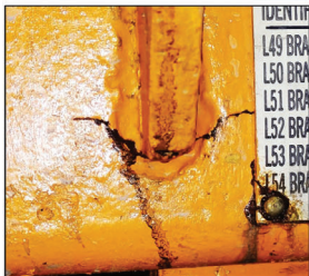
Cracked structural steel
